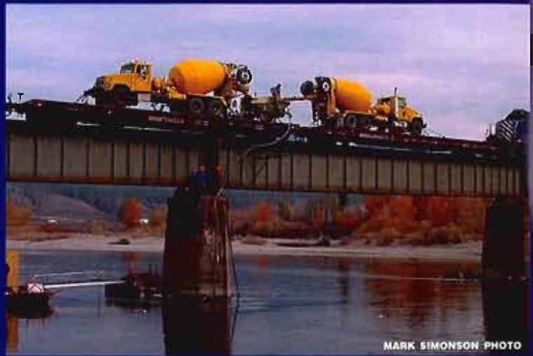
An undermining problem with Pier B on Bridge 141 across the Clark Fork River near Huson, MT was solved with the placement of over 30 yards of a special type of concrete. Aided by MRL B&B Crews 101802 and 101804, underwater divers from Norwesco Marine in Spokane, WA accomplished the repairs on October 26, 2000.
