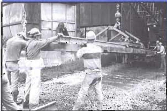
The final track panel being placed on July 19. Photo by Dave Cook.
