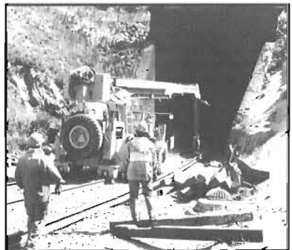
Welded rail being positioned for relaying at the west portal of the tunnel.
