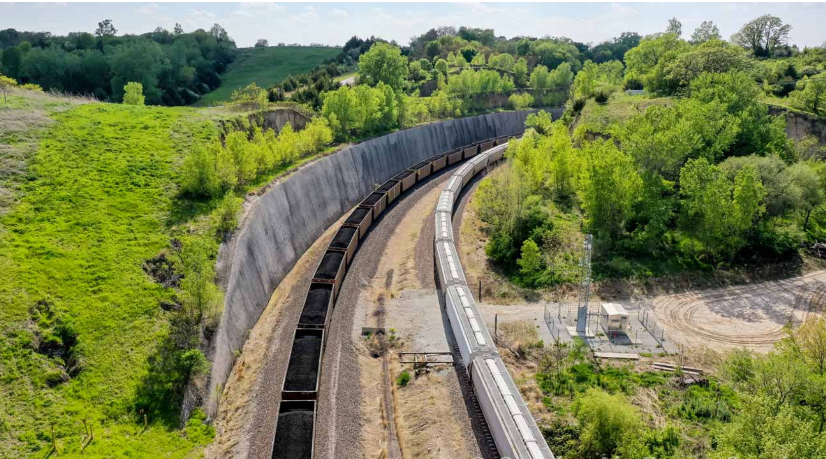
The expanded cut with the second track and the soil-nail retaining wall in place to eliminate erosion problems. A westbound freight awaits passage of an eastbound coal train before continuing on to Lincoln. The dirt road on the right is part of the original line that avoided the bluff. May 5, 2021. Drone photo by Patrick Jones, Omaha Air Drone Service.
